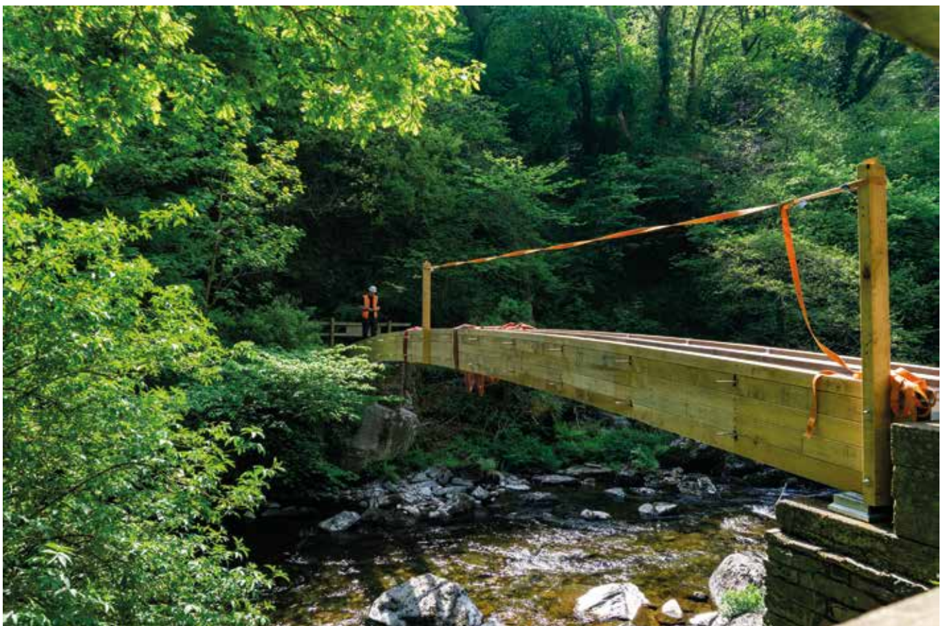
Woodside Bridge, built from oak from conservation management of Burrige Wood. Exmoor National Park, 2020. See Case study 11.
